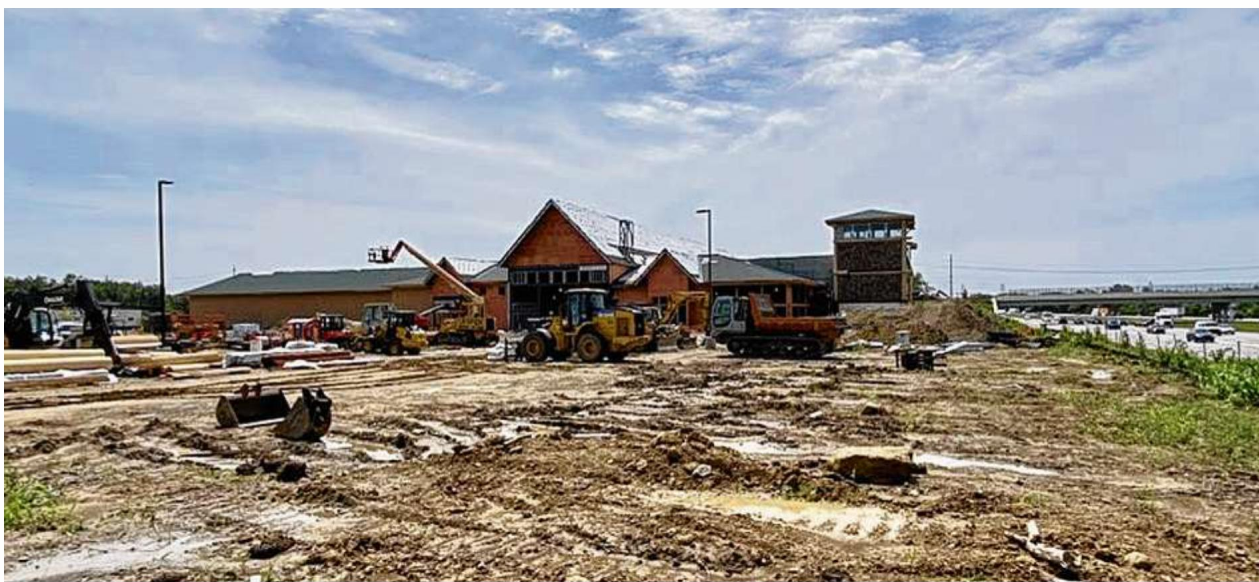
Work continues on the Bass Pro Shop store as seen here Thursday along Interstate 75 North in West Chester Twp. It is expected to open sometime in 2024. MICHAEL D. CLARK / STAFF
